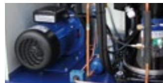
Pump P3 (3 barg) / P5 pump (5 barg, optional).
